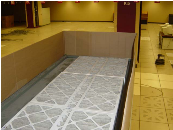
Fig. 3. Cardboard box installed on the top of the A/C unit (filters are covering the air intake of the A/C unit)
